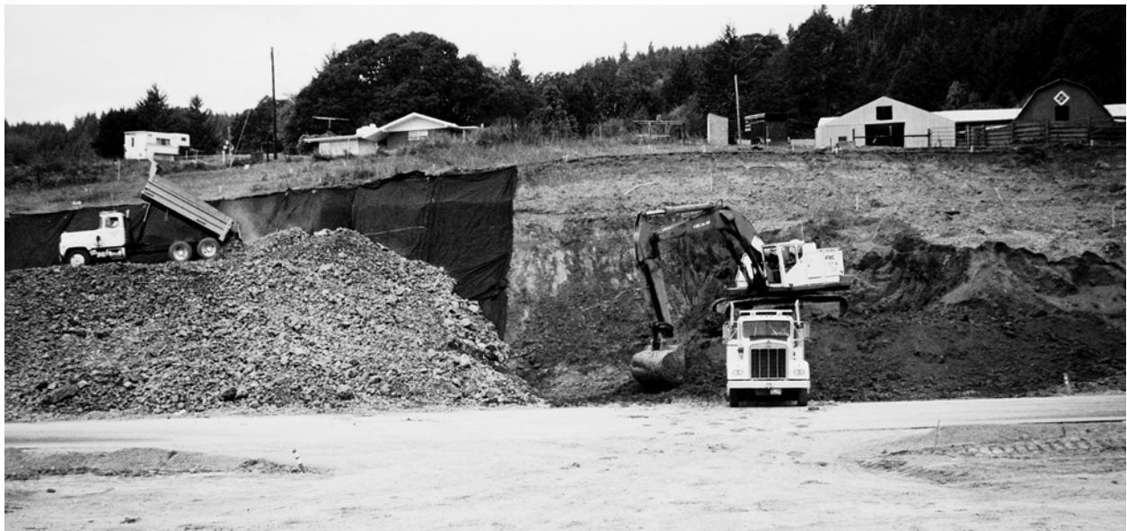
Figure 21. Closely-sequenced construction method being applied at Lorane Road landslide. On right, a backhoe excavates soil and loads spoil into a dump truck. On left, rockfill is being dumped and spread to build a buttress. Filter fabric (dark gray) is laid on the cut slope behind the rockfill.
